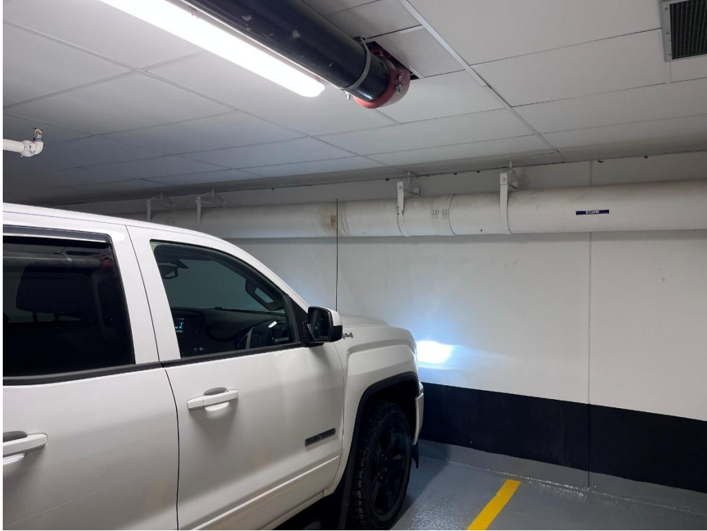
Photograph 4 – showing a Fernbrook truck parking at the building wall which is 5.8 metres from the ‘front’ of the parking space
