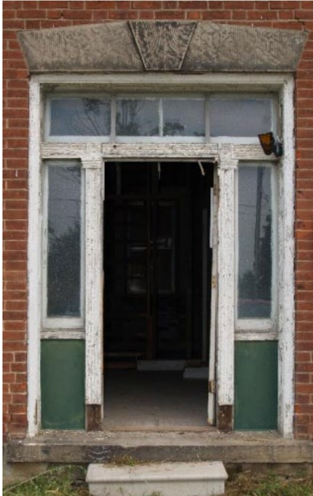
Prior to restoration
