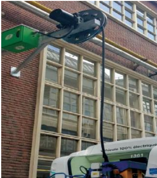
Figure 25. Example of Wall Mounted Cable Reel
