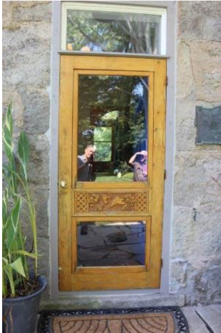
• Front Entrance Door
