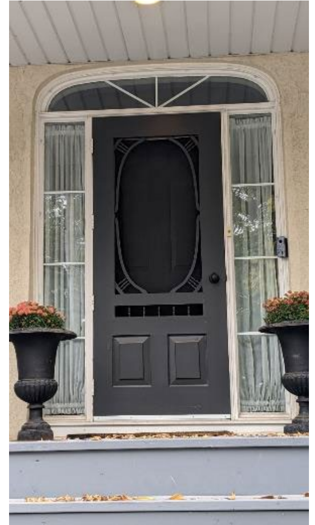
Existing Front Door, single leaf with four panel side lights and elliptical transom
