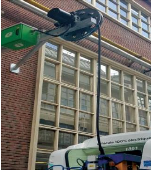
Figure 25. Example of Wall Mounted Cable Reel
