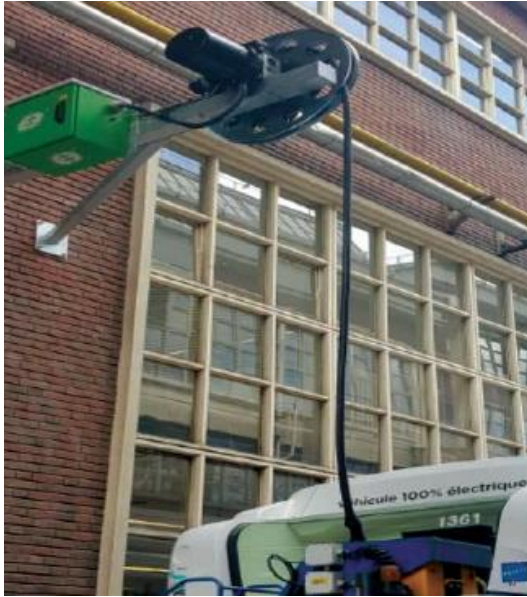
Figure 25. Example of Wall Mounted Cable Reel
