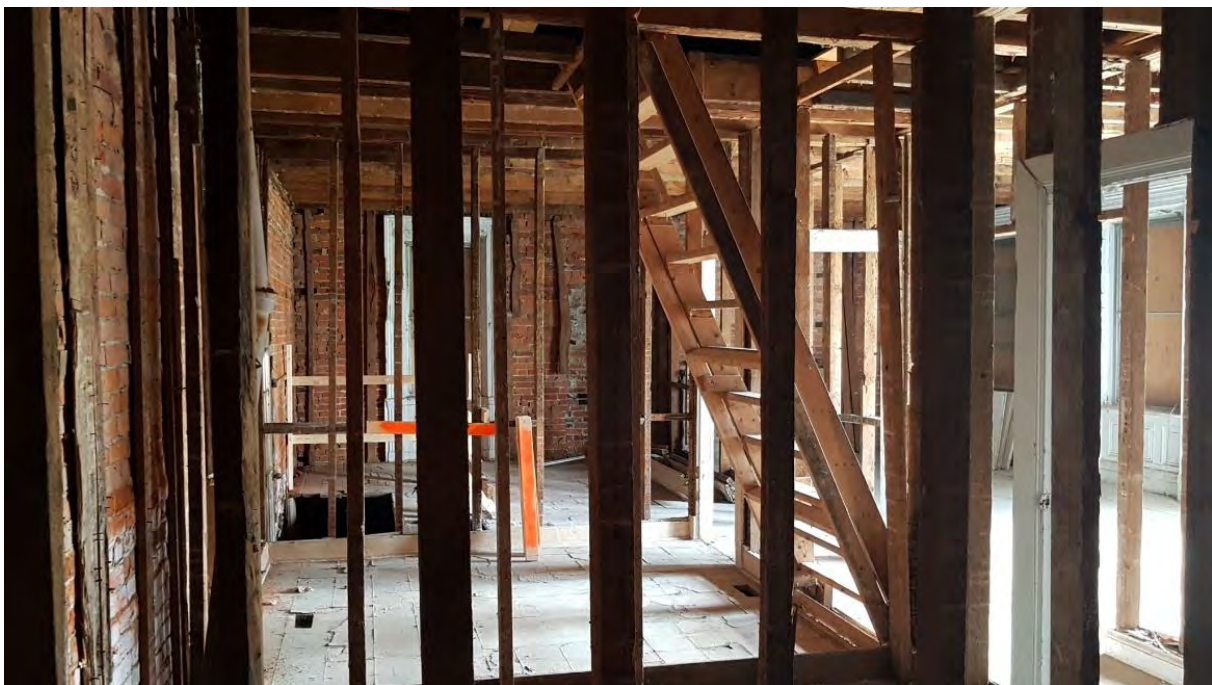
Figure 38: View from one of the bedrooms, showing the washroom, kitchen, another bedroom, and stairs to the attic (August 2018)
