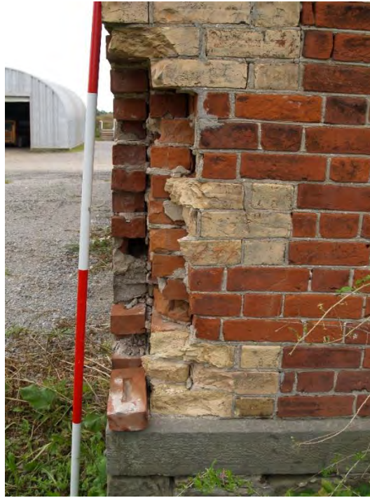
Figure 42: Spalling brick at the corners of Beaty House.
