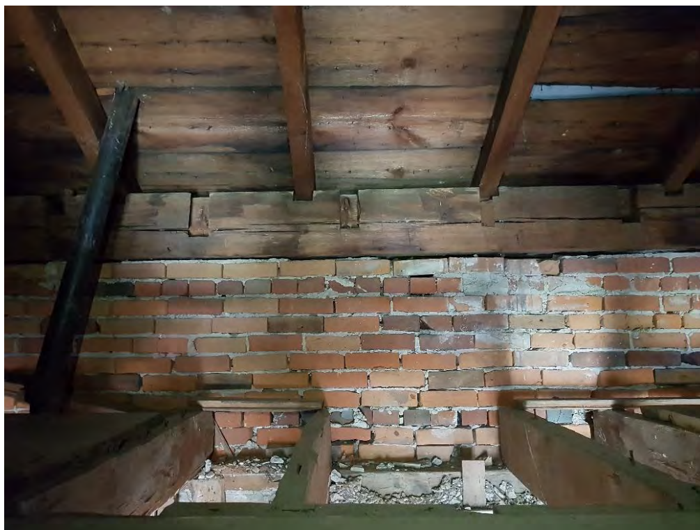
Figure 40: Redundant mortices in wood beams of roof.
