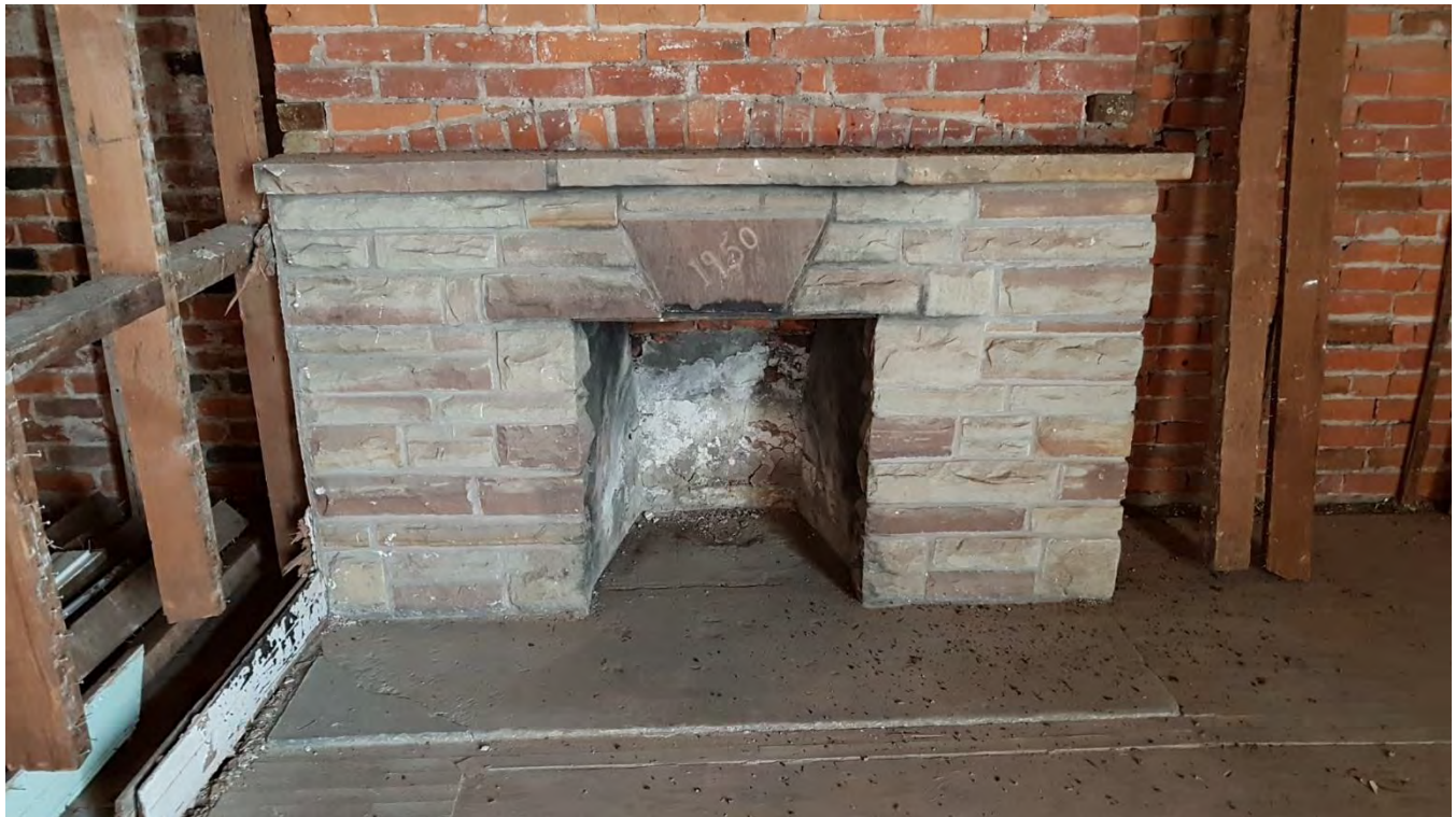
Figure 33: Fireplace on south end wall with 1950 datestone on the stone veneer (August 2018)
