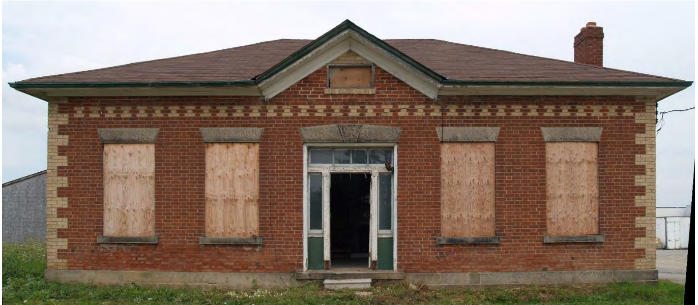
Figure 6: West or principal façade of the Beaty House (August 2018, corrected for distortion)
