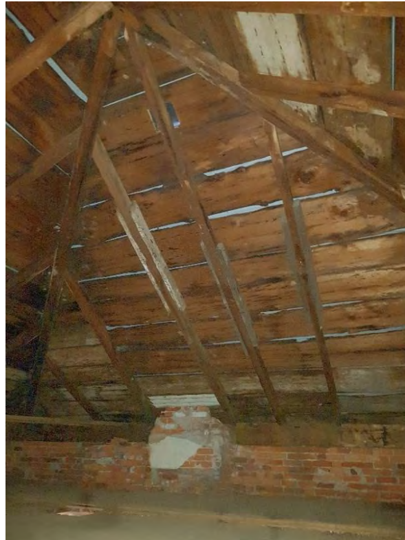
Figure 43: Lack of transition between brick and wood roof from the interior of the attic (August 2018)
