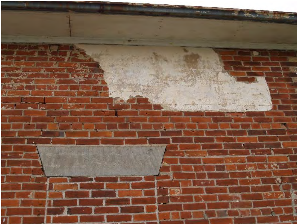
Figure 19: Plaster adhering to the northeast portion of east façade (August 2018)
