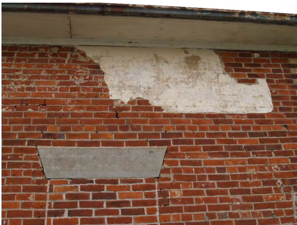
Figure 18: Plaster evident on the north portion of east façade of Beaty House.
