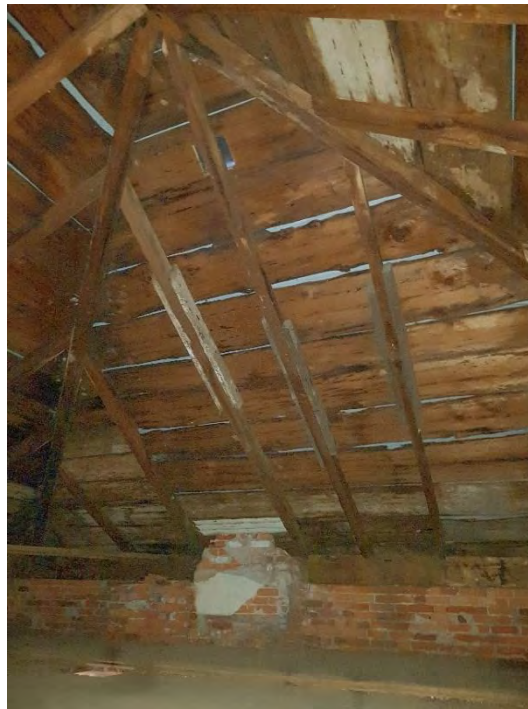
Figure 41: Lack of transition between brick and wood roof from the interior of the attic.
