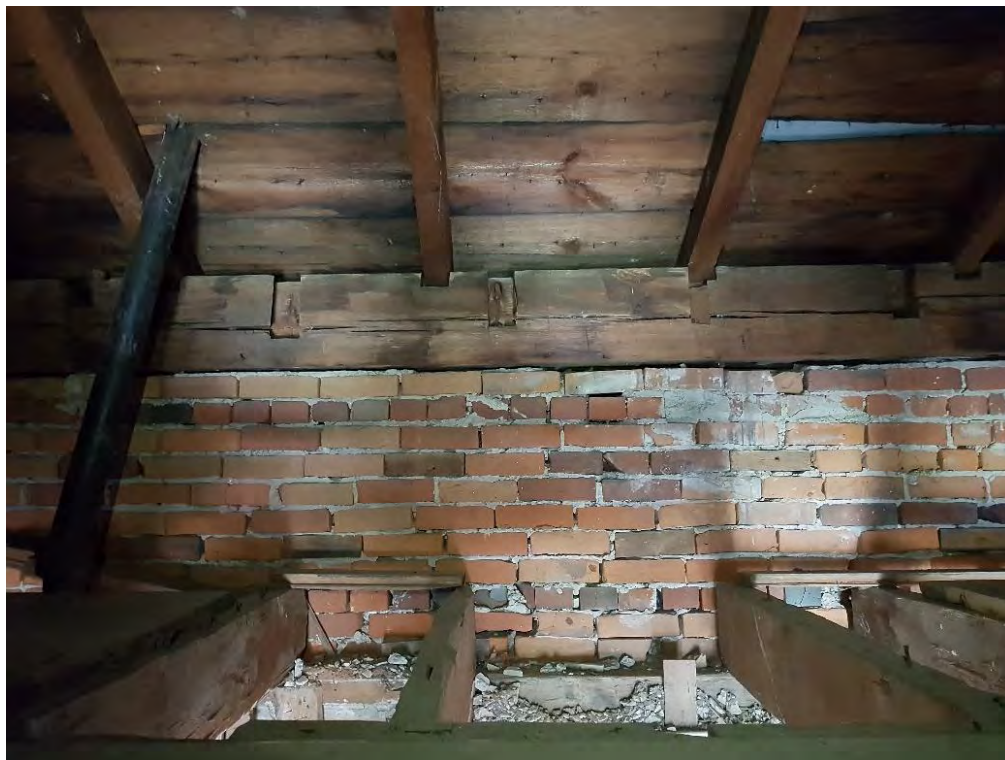
Figure 40: Redundant mortices in wood beams of roof.
