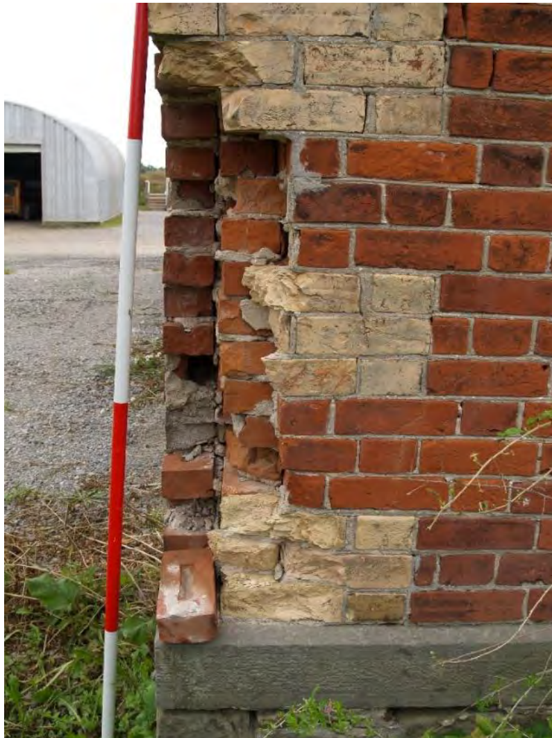
Figure 46: Spalling brick at the northeast corner of Beaty House (August 2018)
