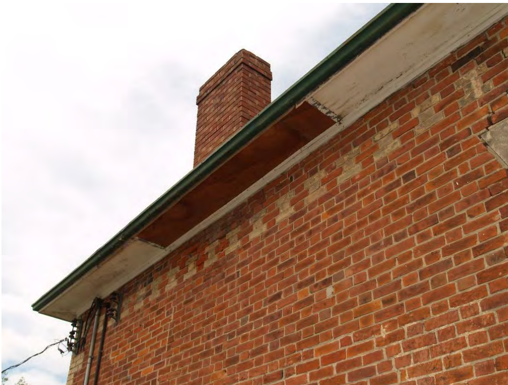
Figure 20: Moulded fascia and soffit on the verges over the south end wall (August 2018)
