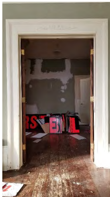
Figure 23: Entrance to the central room from the east room, with decorative wood trim
