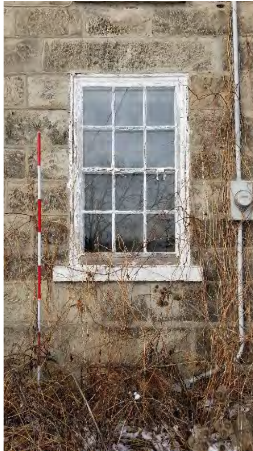
Figure 18: Typical window with stone lintel, plain wood lug sill, and six-over-six window
