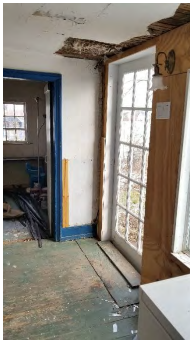
Figure 48: Mudroom facing north towards a closet and an exterior entrance along the east façade
