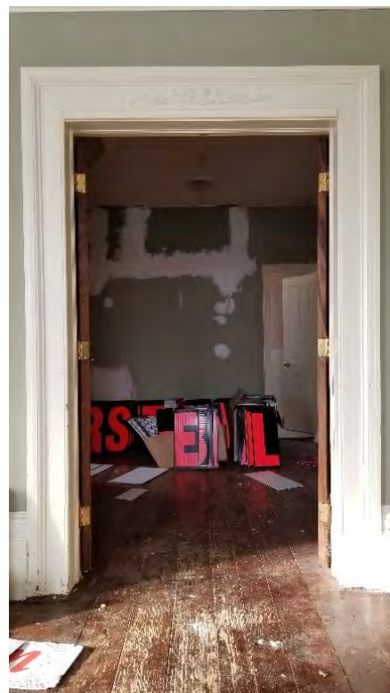
Figure 24: Entrance with wood architrave leading to the central room from the east room
