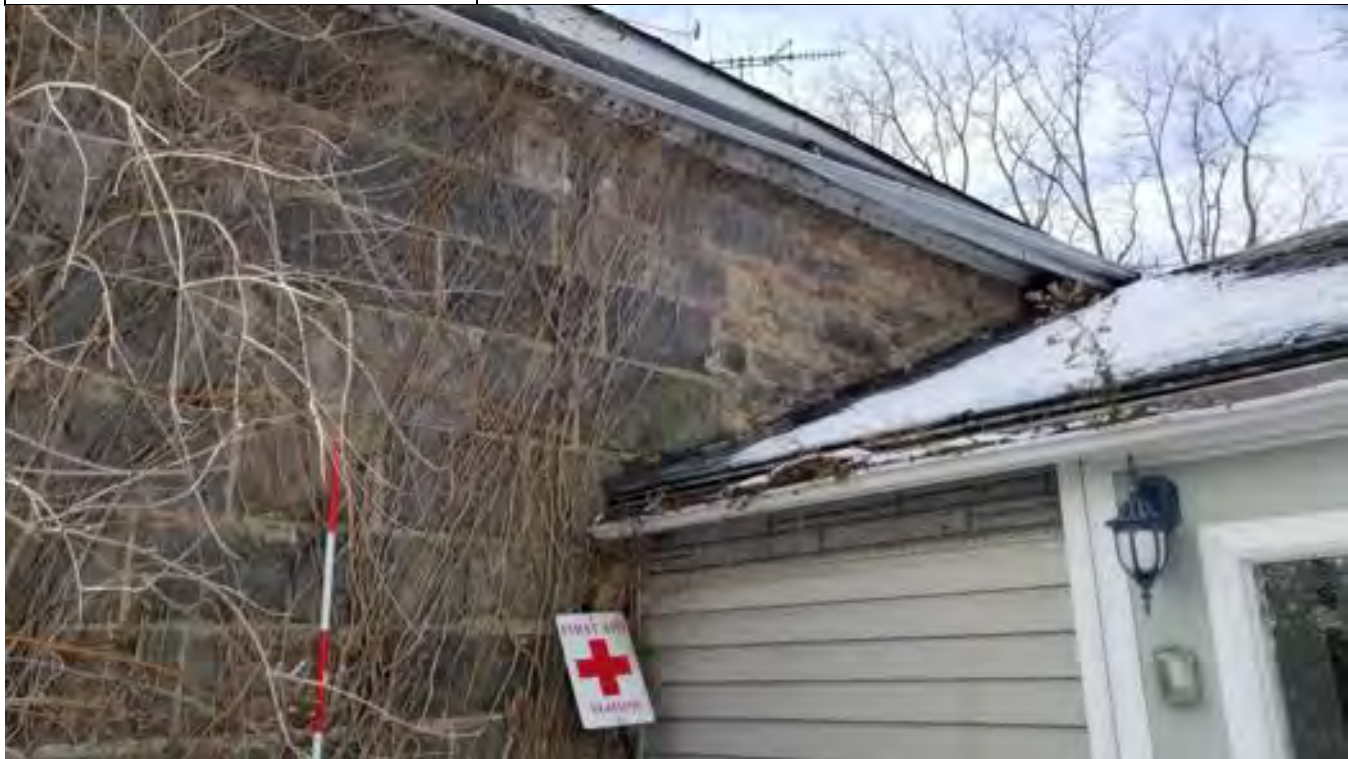
Figure 57: Evidence of cracking on the north facade wall of the Main Block
