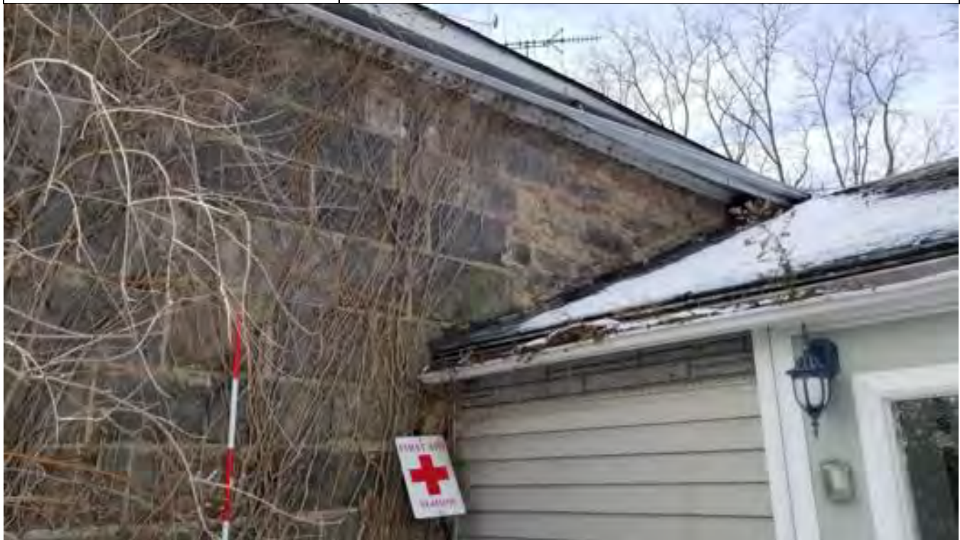
Figure 57: Evidence of cracking on the north facade wall of the Main Block
