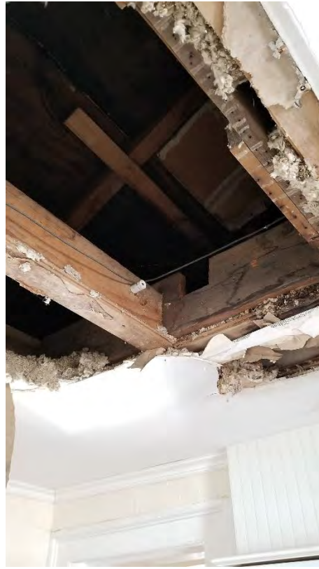
Figure 58: A portion of the collapsed ceiling in the extension kitchen
