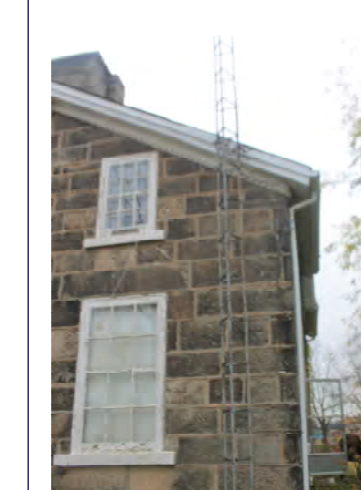
FULL DETAIL AND DIMENSION SHALL BE NOTED ON HISTORIC FLUE PRIOR TO DISMANTLE
