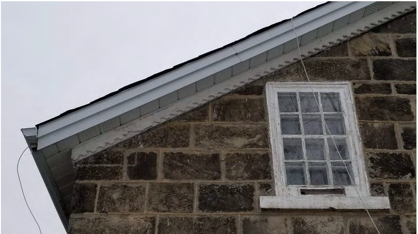
Figure 16: Projecting eaves and verges with plain fascia, metal soffit, and nebulé or nebulé moulding on the frieze
