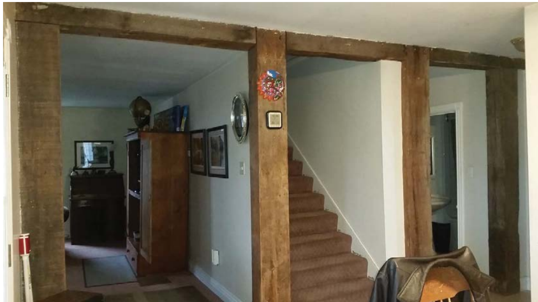
Figure 29: Exposed timber framing on the north wall of the main block. The load bearing posts of two bents are either side of the stairs, while at each end are non-load bearing vertical studs. Three cross braces run across the ceiling.
