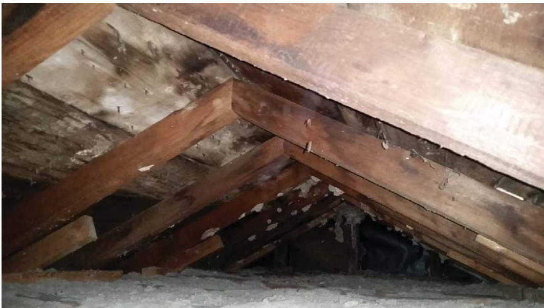
Figure 54: Roof construction of the main block as seen from the attic access.
