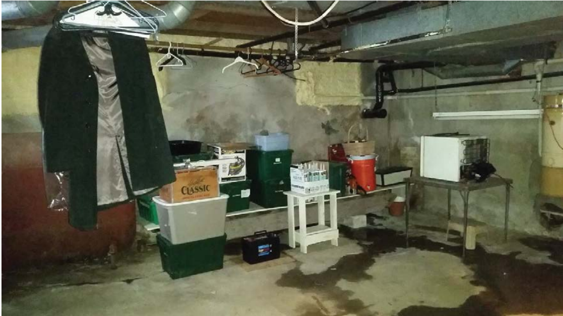
Figure 51: Portland cement parging and poured concrete floor in the main block basement.
