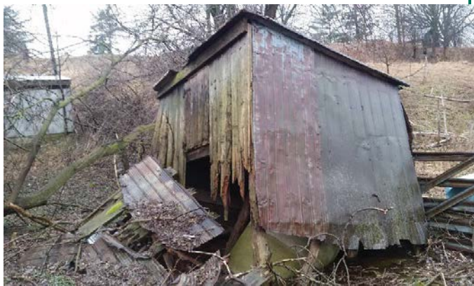
Late 20 th century shed (left) and partially collapsed wood plank shed (right)
